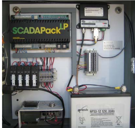
Figure 2 – Typical Telemetry Site Equipment
