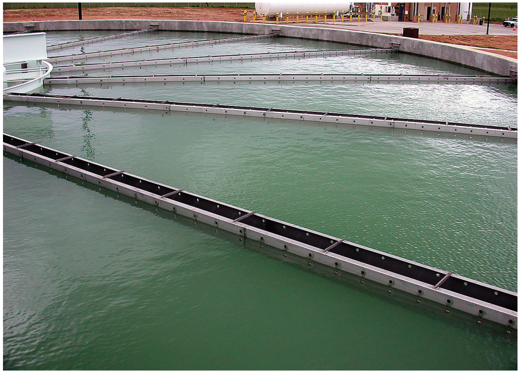
Figure 10-3. Clarification, second step of treatment process.
