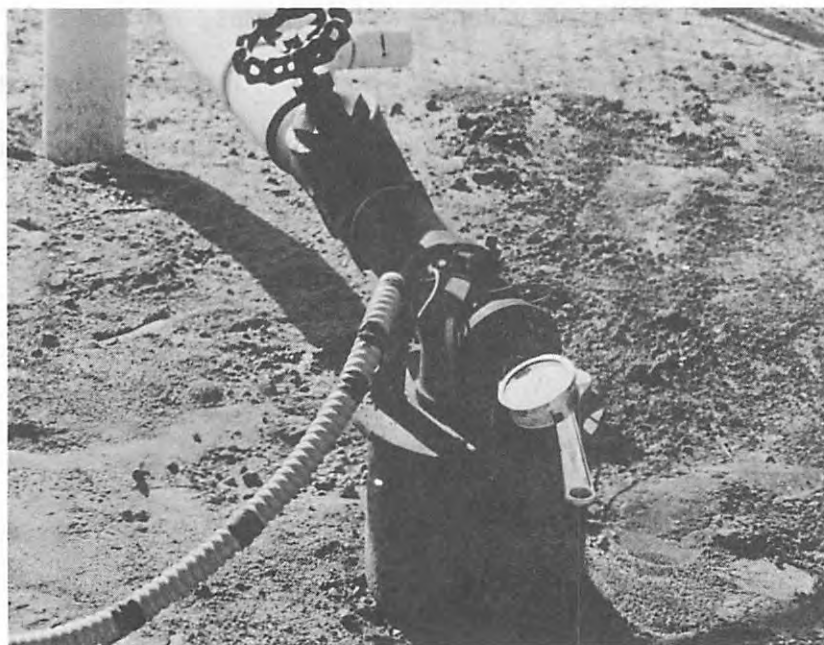
The pressure is being checked to find the additional work required by the pump above the pump lift.
