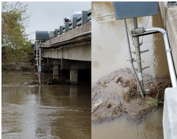
Figure 12. Damage resulting from Hurricane Harvey at USGS station 08188810 Guadalupe River at SH 35 near Tivoli, Tex.
