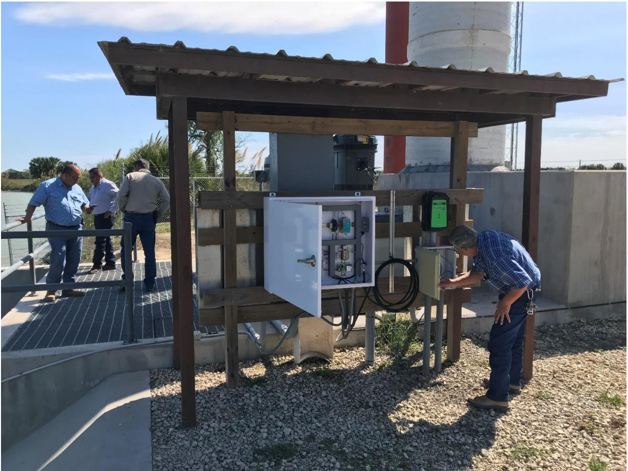
Figure 25 Unit 8 SCADA System panel and flow meter.
