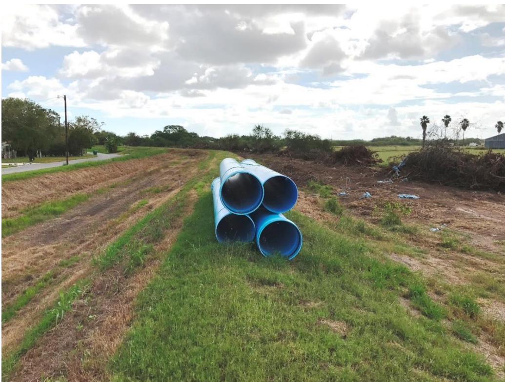
Figure 10 Photo, 7.25.16, clearing for the new pipeline. Pipe materials on site. Note the large open canal that is being replaced.
