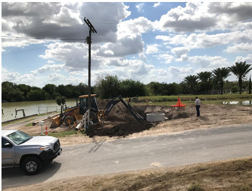
Figure 17 Photo, 10.27.17, District working on connection of new Resaca crossing to upstream Saldaña Canal.
