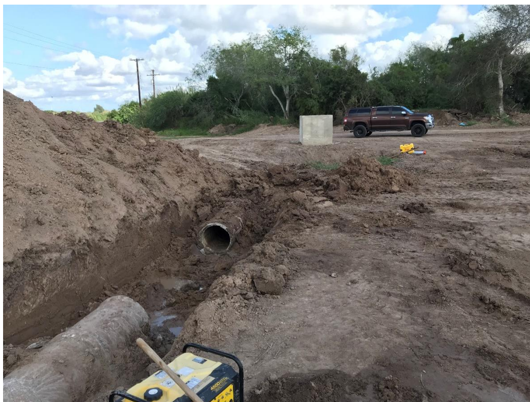
Figure 18 Photo, 11.17.17, District working on connection of existing lateral to new Saldaña Canal.
