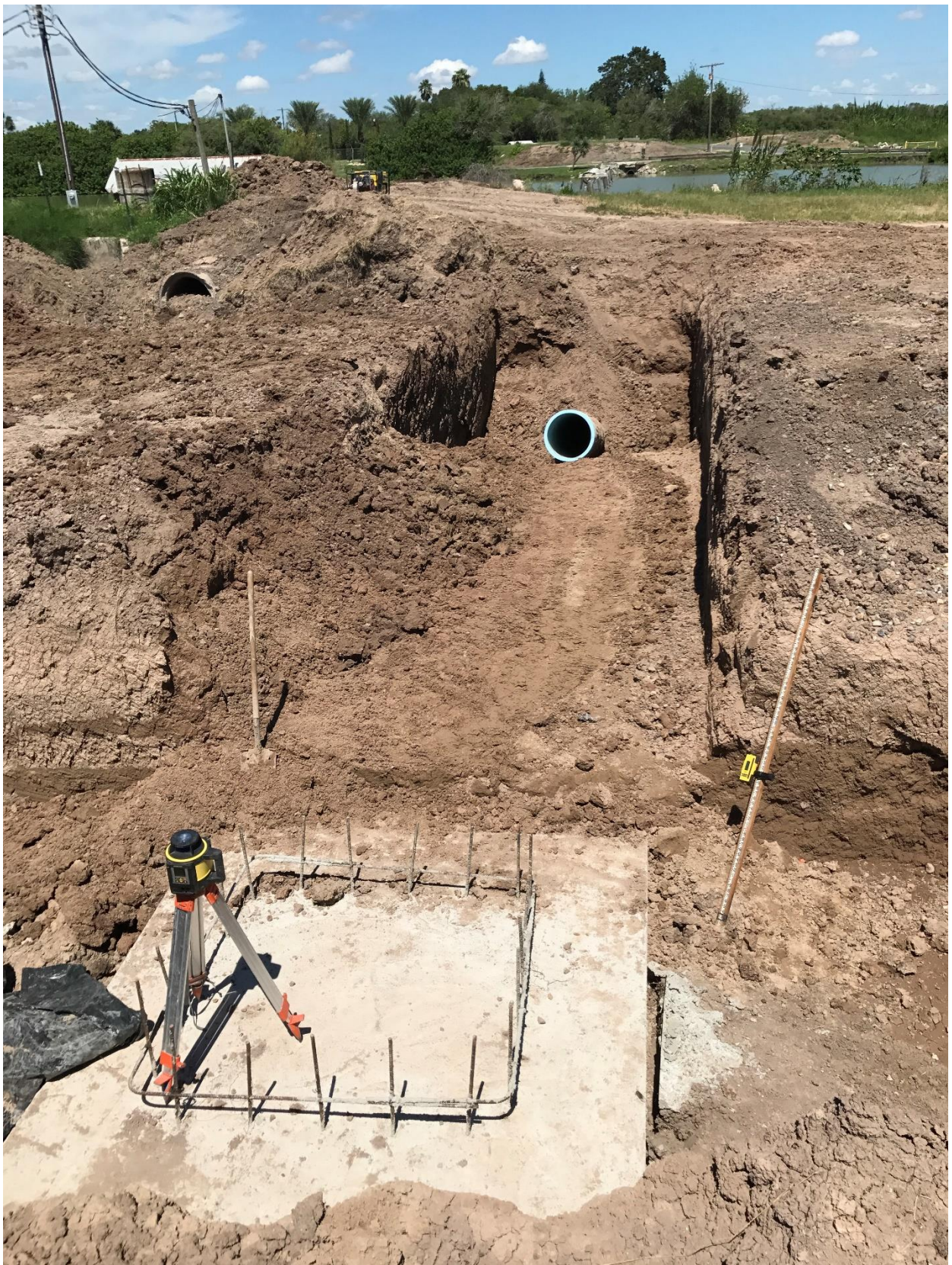
Figure 16 Photo, 8.29.17, foundation for well at station 0+73, prepared for well construction. 24 inch fused PVC directionally drilled under Resaca in background.
