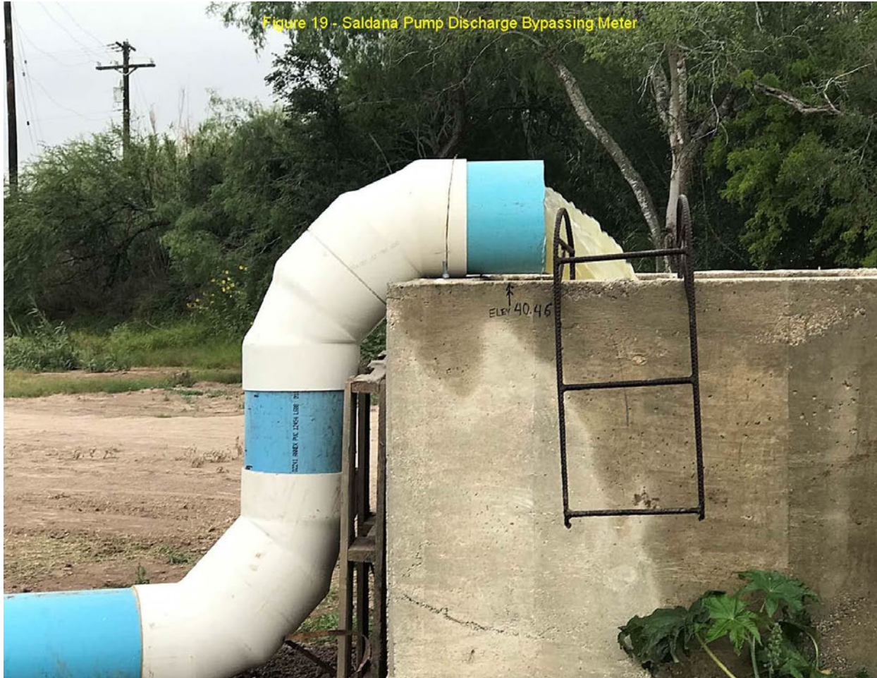
Figure 19 Saldaña Pump Discharge Bypassing Meter
