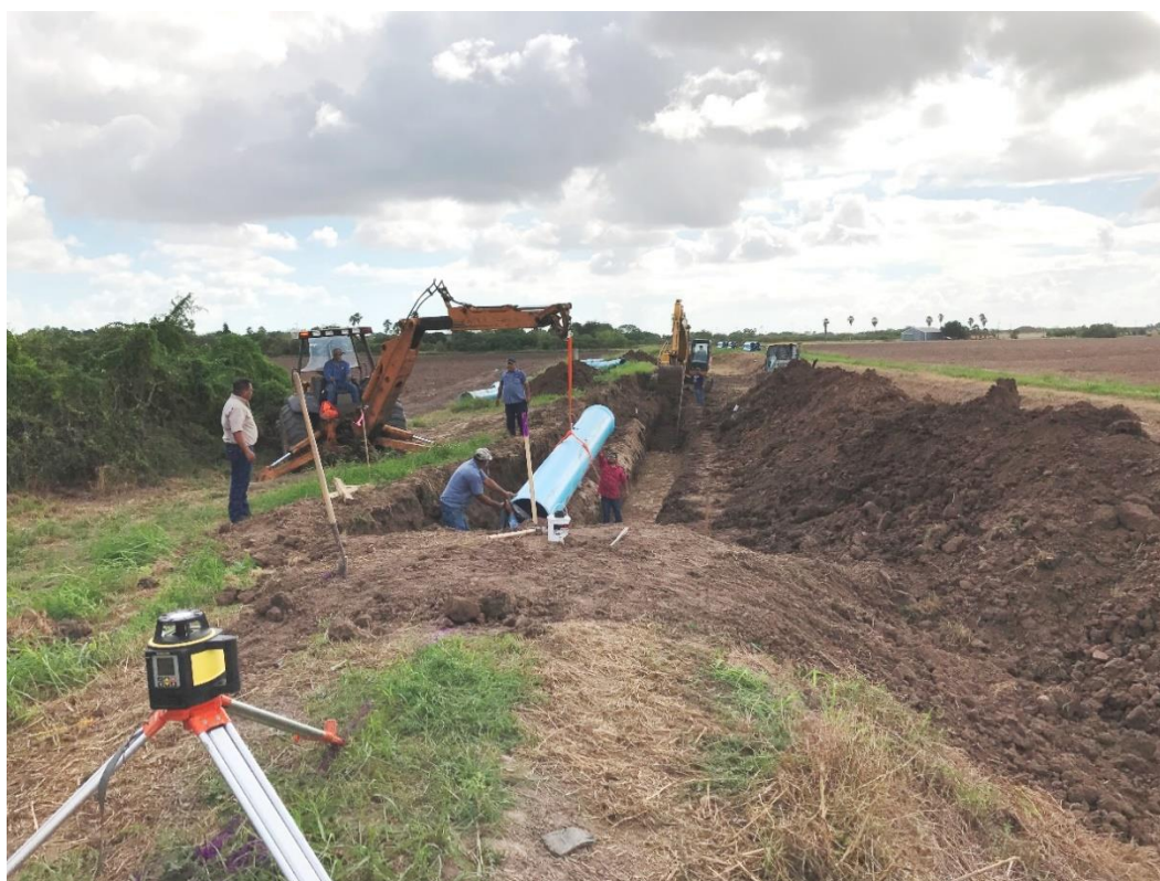
Figure 11 Photo, 11.2.16, laying new PVC pipeline. New PVC pipeline to replace the open canal.
