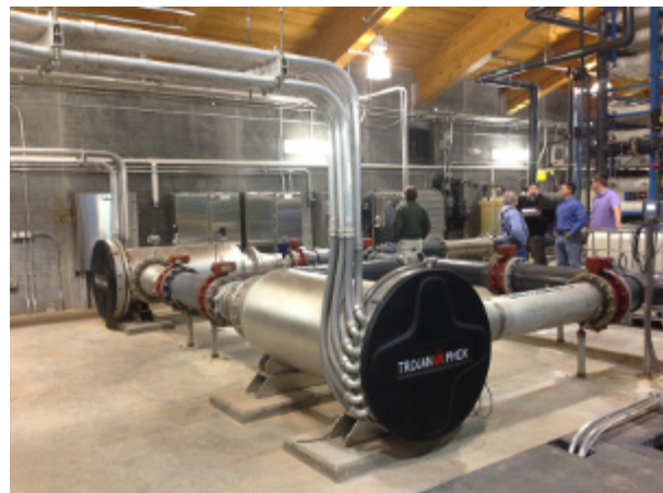
UV Reactors at the Raw Water Production Facility Photo Credit: Eva Steinle-Darling
