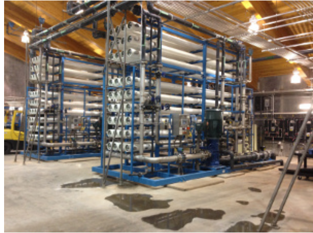
RO Skids at the Raw Water Production Facility Photo Credit: Eva Steinle-Darling
