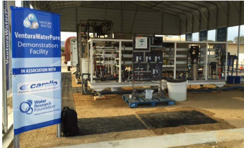
Reverse Osmosis Skid at VenturaWaterPure Demonstration Facility Photo Credit: Justin Sutherland
