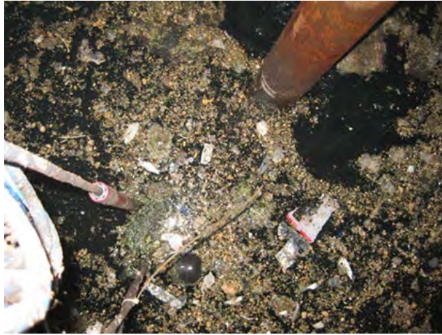
Figure 5-5: Existing reclaimed water wet well (photo by Terry Mitchell, 2011).
