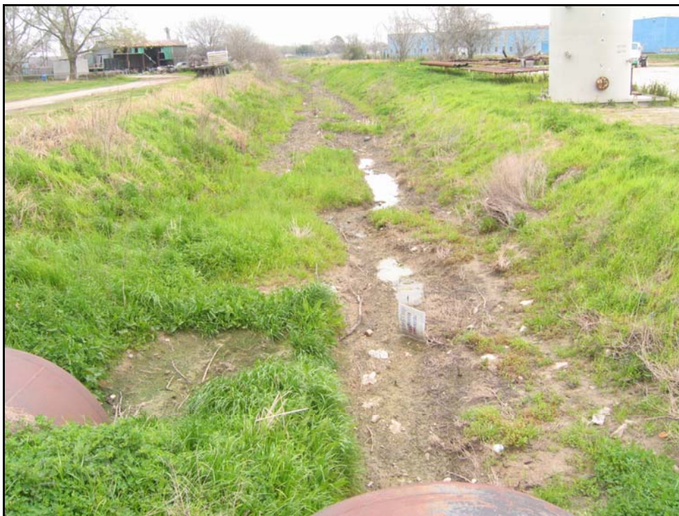
Figure D8: Sediment in channel downstream of South Meadow Lane
