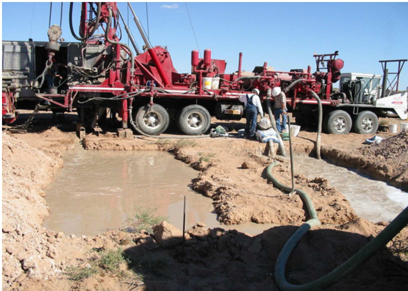
← c. DRILLING MUD CIRCULATION PITS
