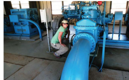
Sampling at Moss Creek Lake Pump Station
