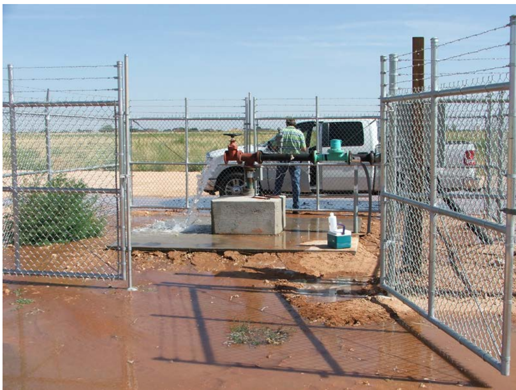
Figure 1. Santa Rosa Well during purge before sample collection, August 1, 2012
