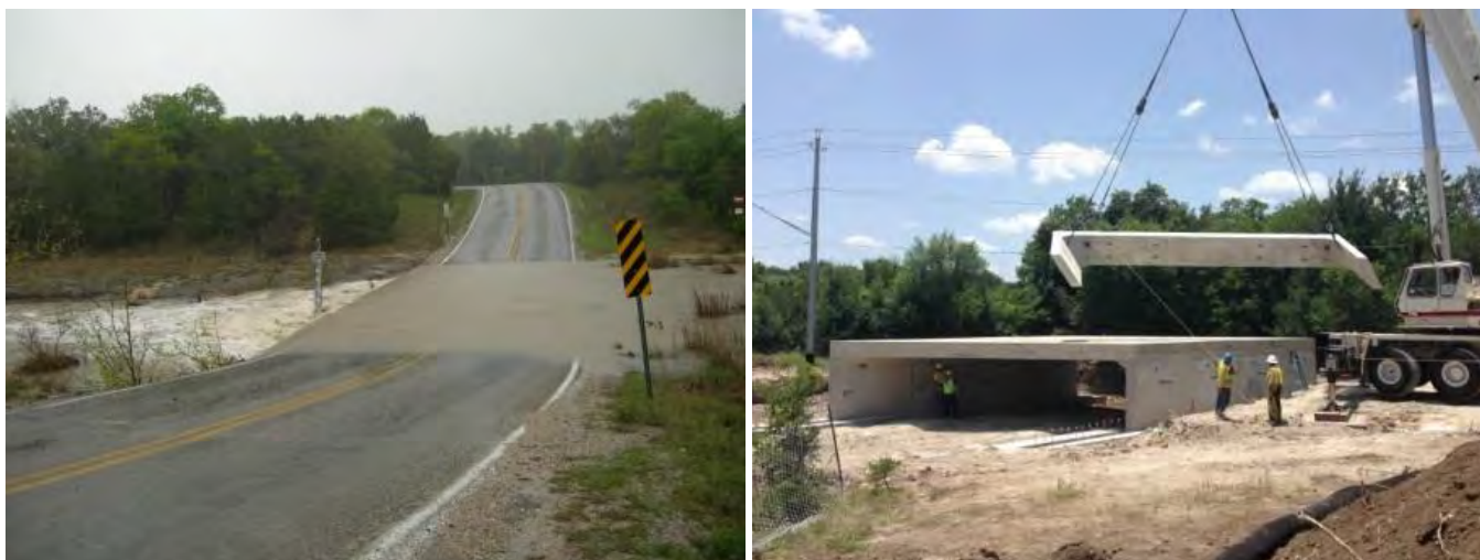
Example of Flooded Low Water Crossing at Bee Creek Road and Bee Creek in Travis County as well as an Example Low Water Crossing Upgrade with Precast Bridge Units, David Moore Drive, Austin
