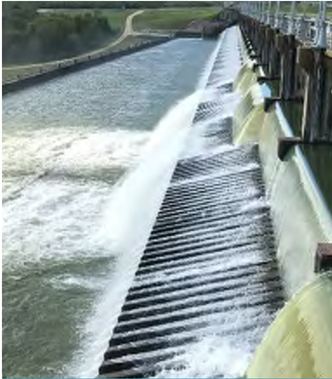
Flood gates at Lake Corpus Christi, May 2019
