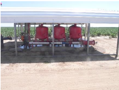
SDI Drip station
