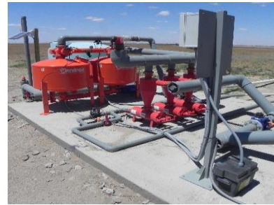
SDI filtration system
