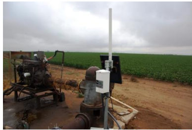
Surface turbine irrigation well
