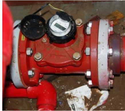
Meter on SDI drip system
