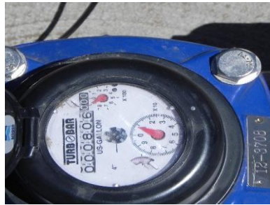
Water meter on system
